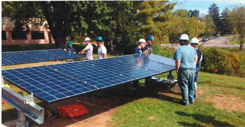
Mid-State Technical College and Pittsville students install a photovoltaic system at Pittsville High School. (Digitized photo)
